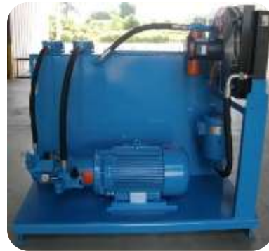
50 HP BOOSTER PUMP
