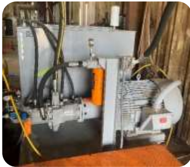
100 HP INJECTION BOOSTER PUMP
