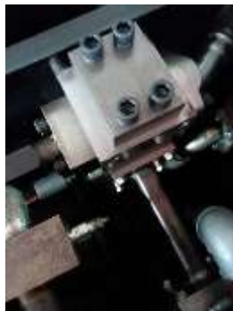
JUNCTION MANIFOLD INSIDE HYD. TANK
