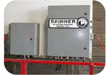
PLC & VFD DRIVE PANELS
